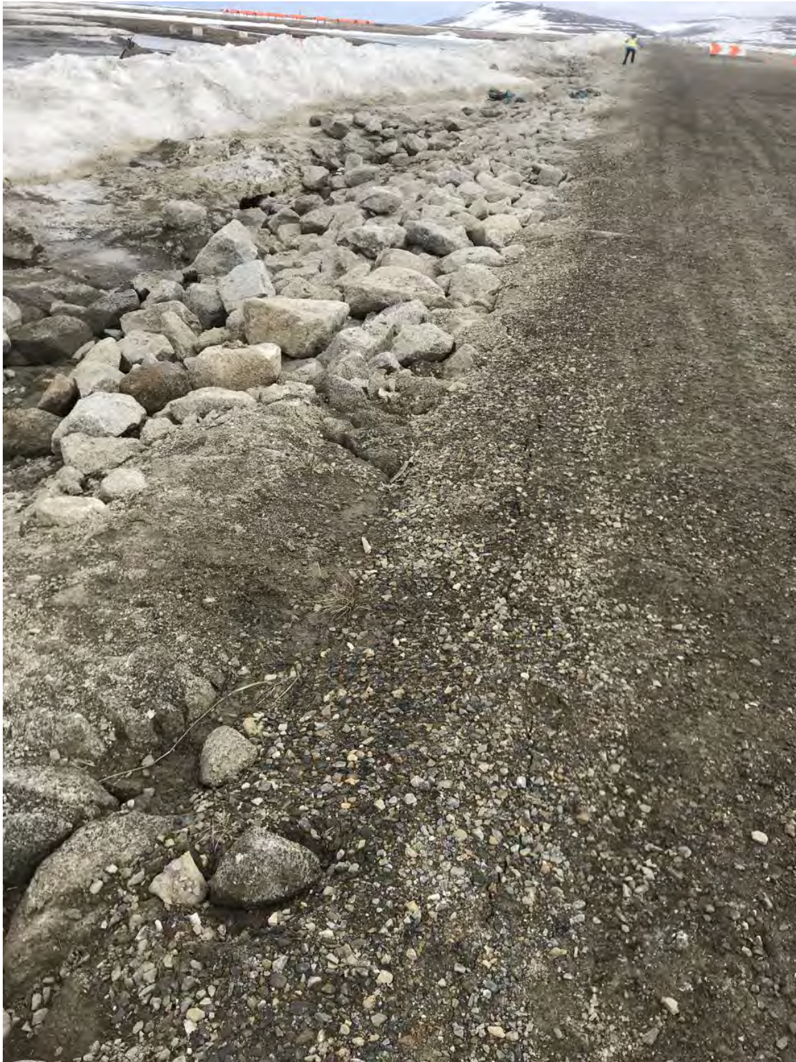
Figure 12. Armor rock protection at western terminal along north edge (looking east). Some rocks observed to be displaced but less than at the western end.
