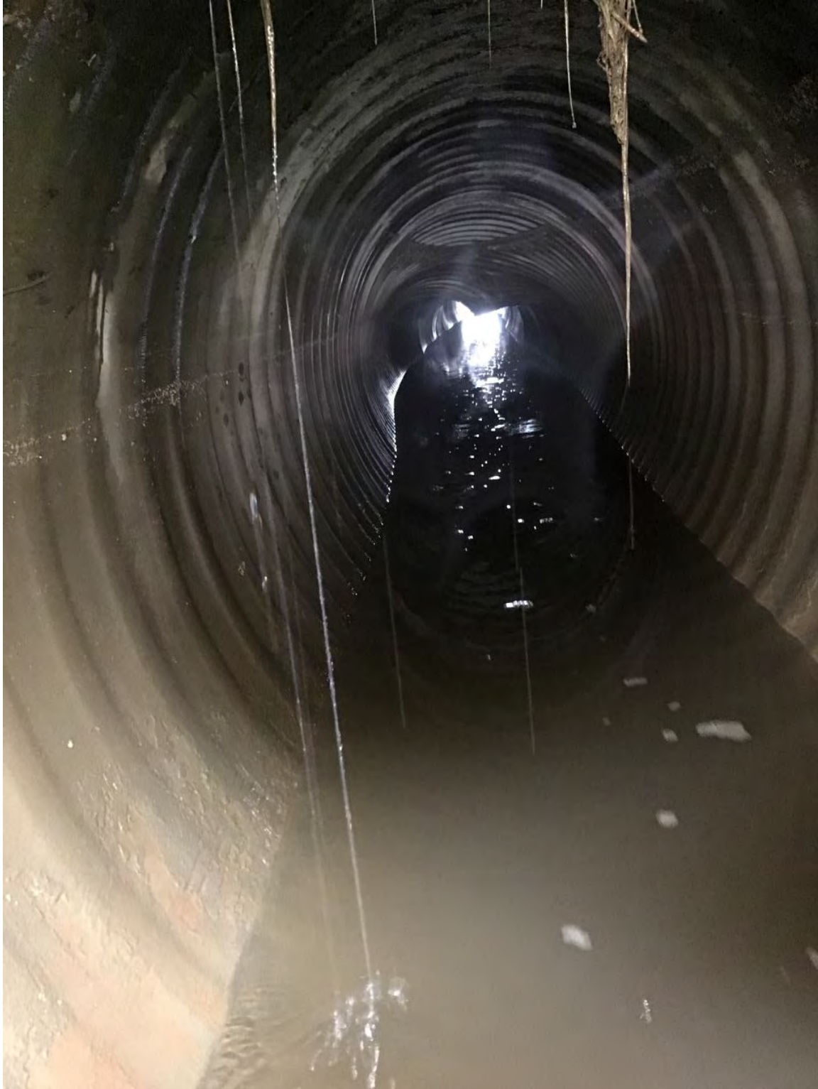
Figure 6. Inside runway culvert looking from outlet to inlet. The culvert was observed to have some sagging and partially collapse in three locations
