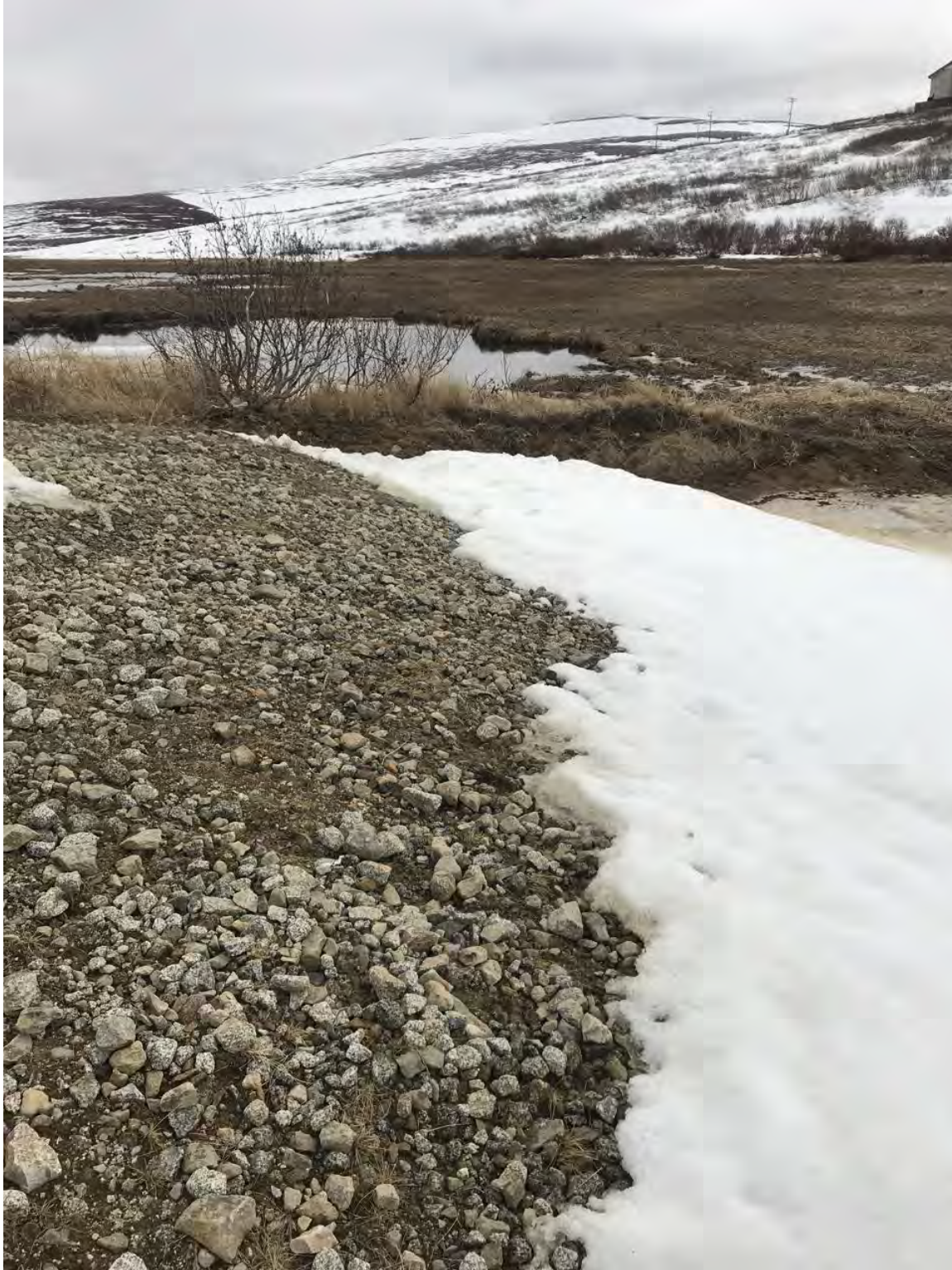
Figure 8. Side slope at windsock (closest point to adjacent elevation). No obvious scour or erosion caused by storm surge/waves.
