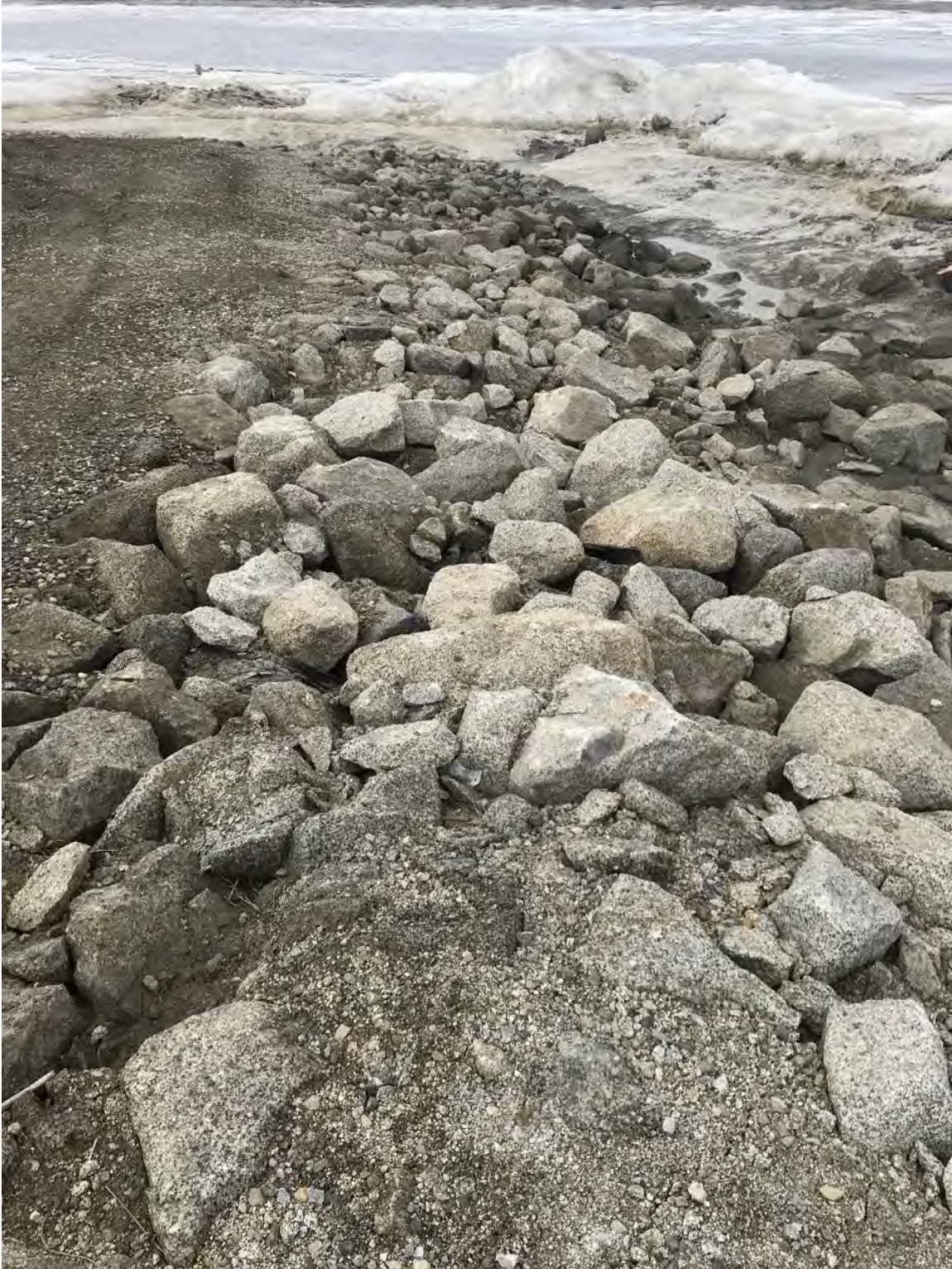
Figure 11. Armor rock protection at western terminal along north edge (looking west). Some rocks observed to be displaced.
