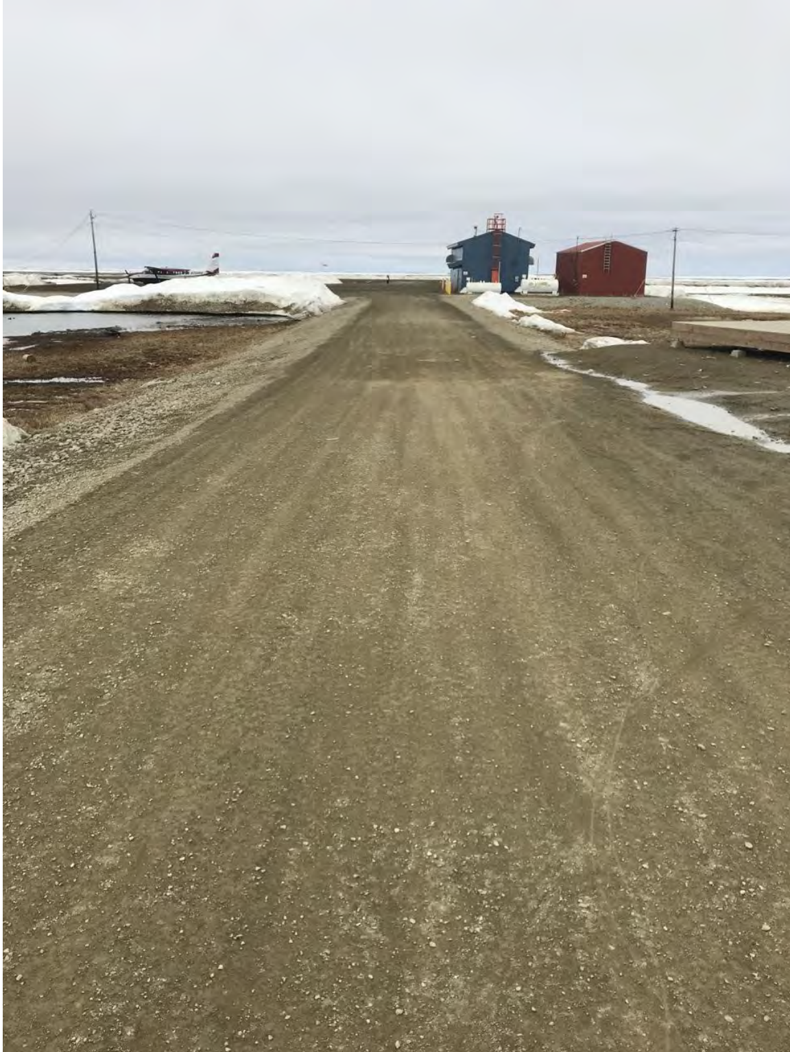
Figure 1. Runway access road. Side slopes appeared to be in good condition – no obvious signs of scour/erosion.
